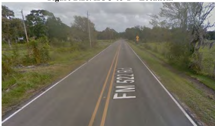
Figure B.29. HOU-03-2 - Asphalt pavement with ACP Overlay. (Source: Google)
